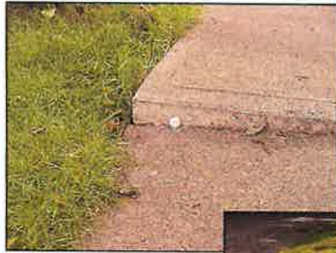
EXAMPLE: 3/4 INCH TRIP HAZARD
