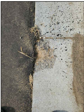
DAMAGE WITH AGGREGATES EXPOSED
