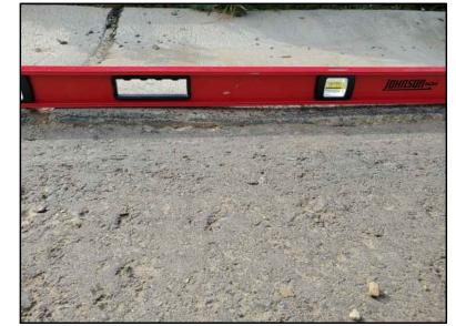
UNEVEN GRADE PLACEMENT/UNEVEN TOP OF GUTTER PLATE
