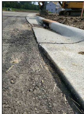
UNEVEN JOINT PLACEMENT/MATCH
