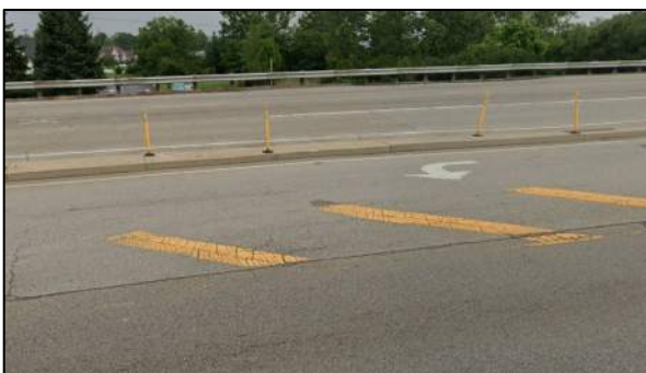
Photo 8: Westbound Left Turn Lane Worn Pavement Markings
