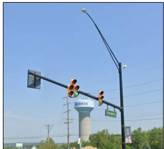
Photo 4: Typical Strain Pole at Main Street Intersection
