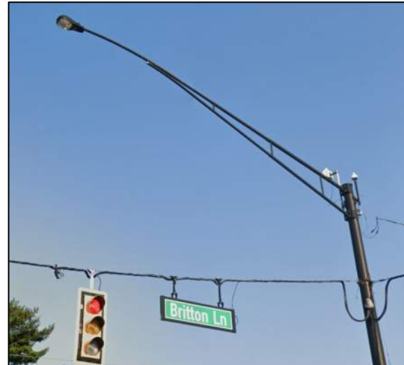
Photo 1: Typical Britton Lane Strain Pole with Luminaire
