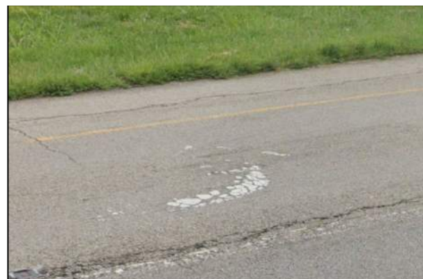
Photo 10: Worn Pavement Markings on Eastbound Left Turn Lane
